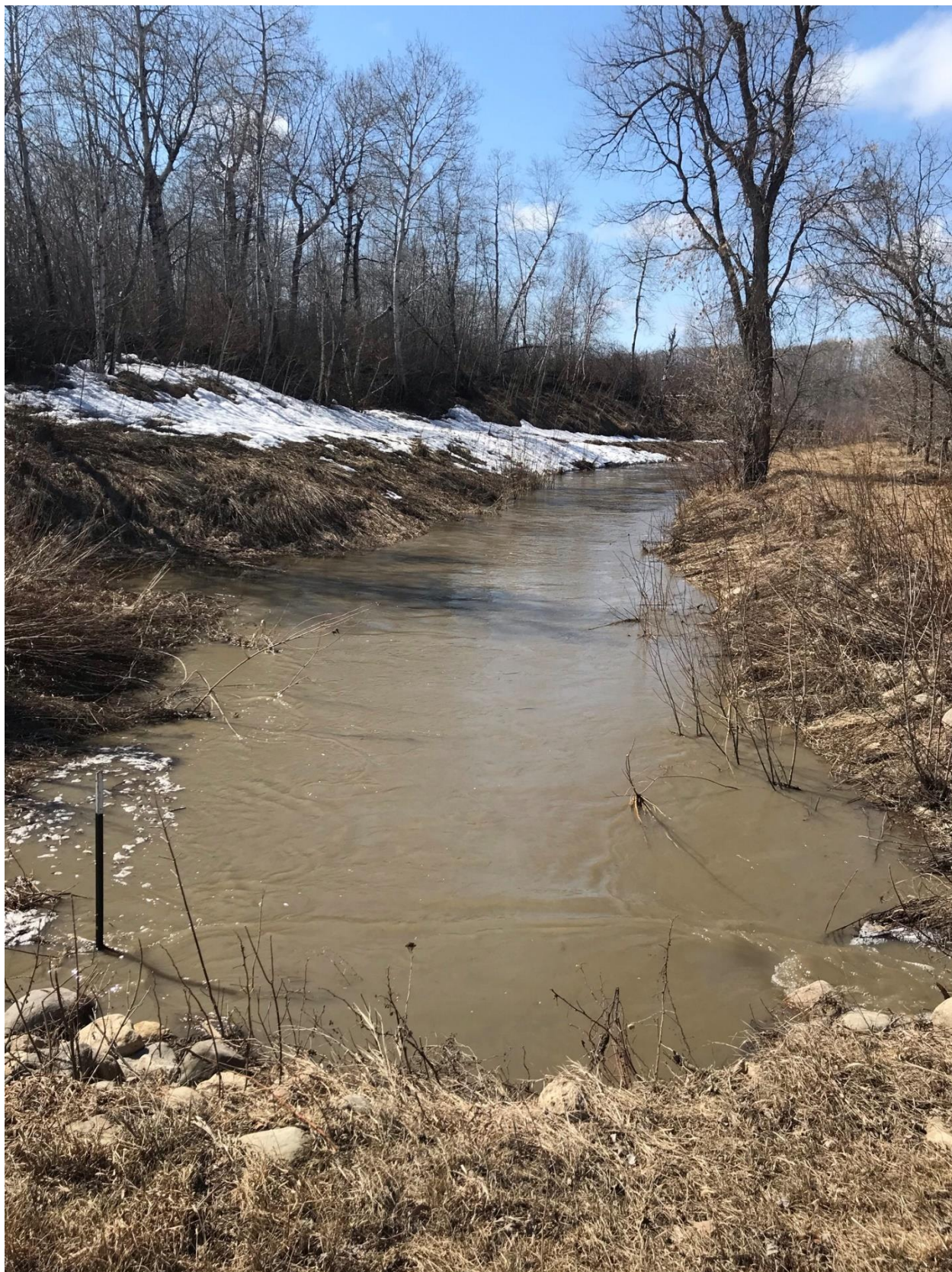
Appendix 7: Culverts not visible - a good indication that velocities are too high to allow fish passage ( >1.5\text{m/s} )
