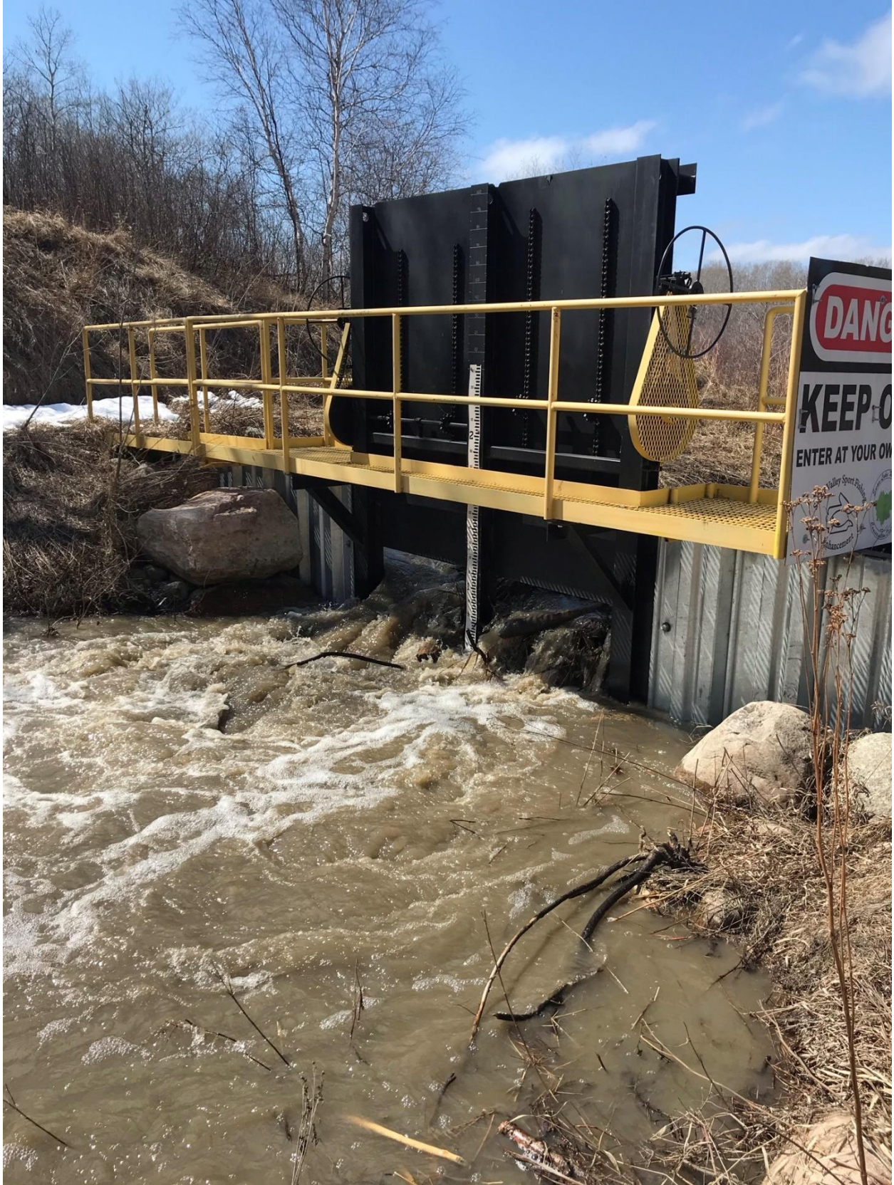
Appendix 2: Control Structure With Debris (May 1, 2022)
